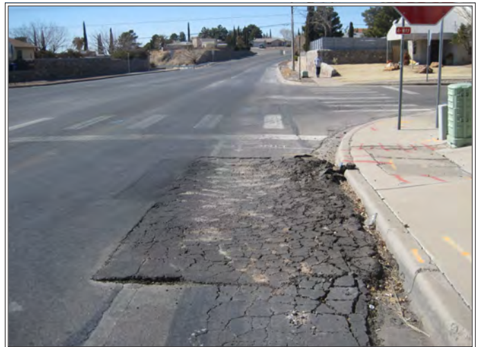
Poor pavement quality is a major safety concern.
